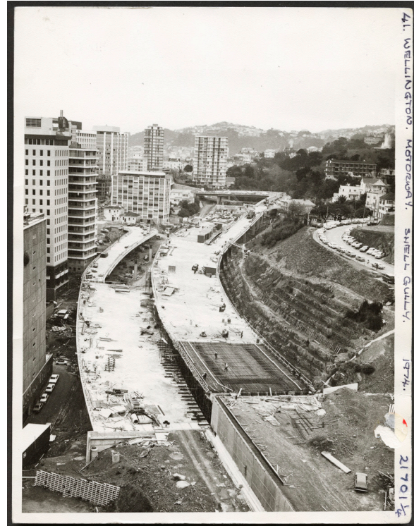
Wellington urban motorway under construction at Shell Gully, c. 7 August 1974, PAColl-9150-24, Alexander Turnbull Library, Wellington, New Zealand.
