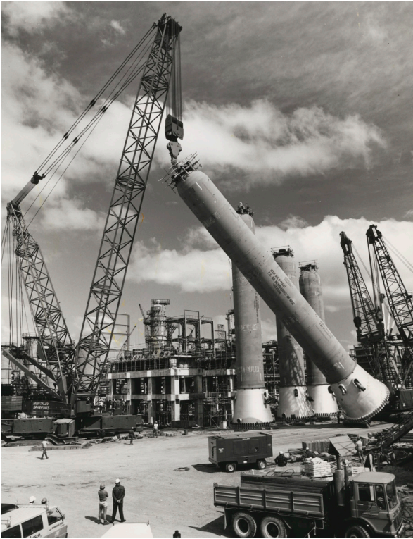
Hydocracker unit reactor lifted by crane, Marsden Point Refinery, 1984, Alexander Turnbull Library, Wellington, New Zealand.
