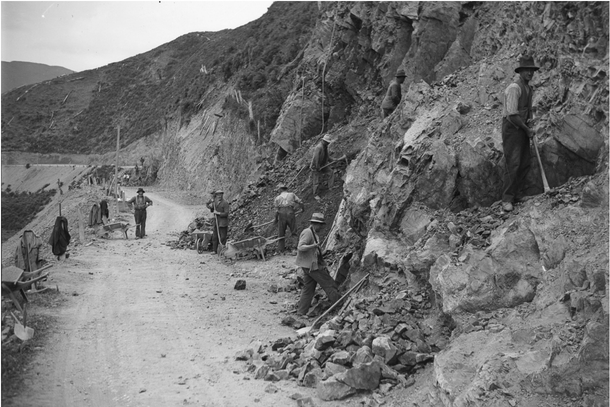
Relief workers excavating the hillside to improve the Akatarawa Road, January 1932, 1/2-084131-G, Alexander Turnbull Library, Wellington, New Zealand.
