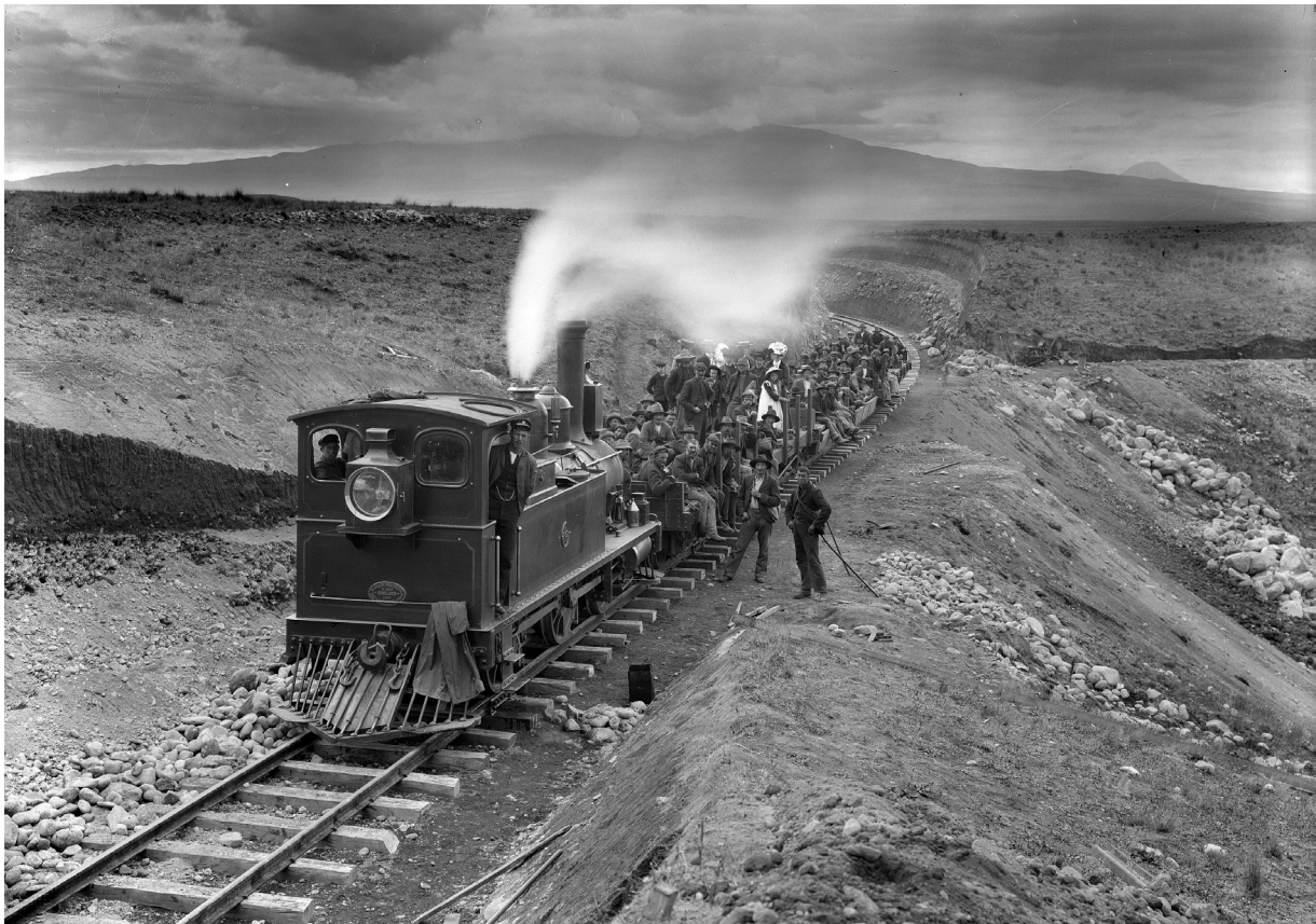
A construction team on the North Island Main Trunk Line, Volcanic Plateau, 1908, 1/1-007689-G, Alexander Turnbull Library, Wellington, New Zealand.
